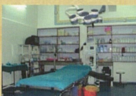
Operation Theatre with Laminar Flow
